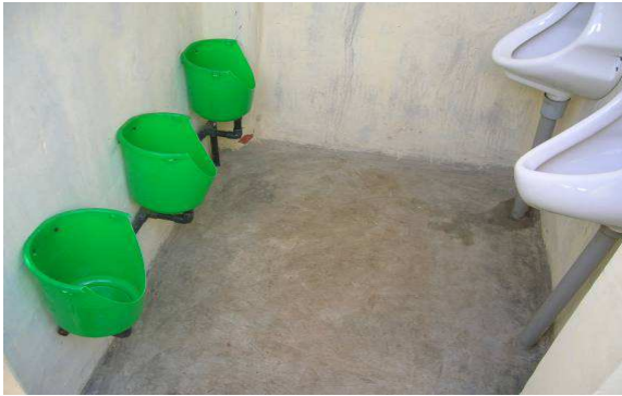
Fig. 7: Inside the men's urinal showing the fabricated plastic containers urinal for the kids and standard ceramic urinals.
